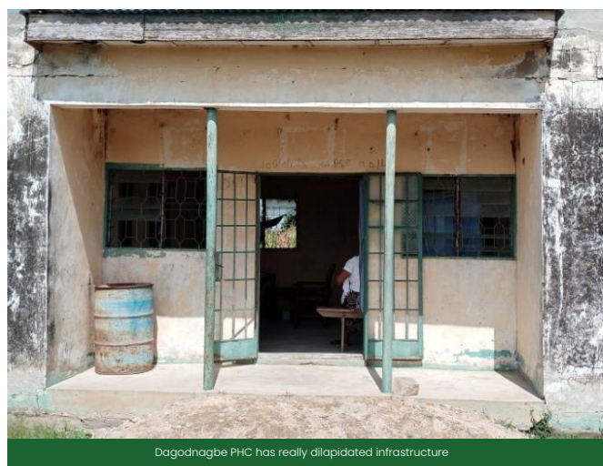
Dagodnagbe PHC has really dilapidated infrastructure
