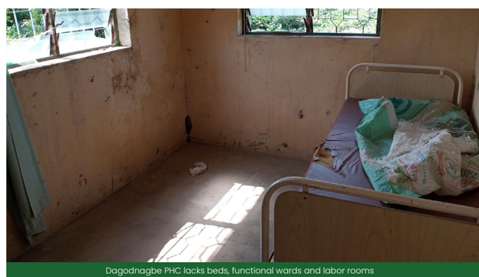
Dagodnagbe PHC lacks beds, functional wards and labor rooms
