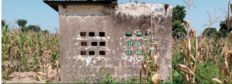
The only toilet at Dagodnagbe PHC is in poor condition
