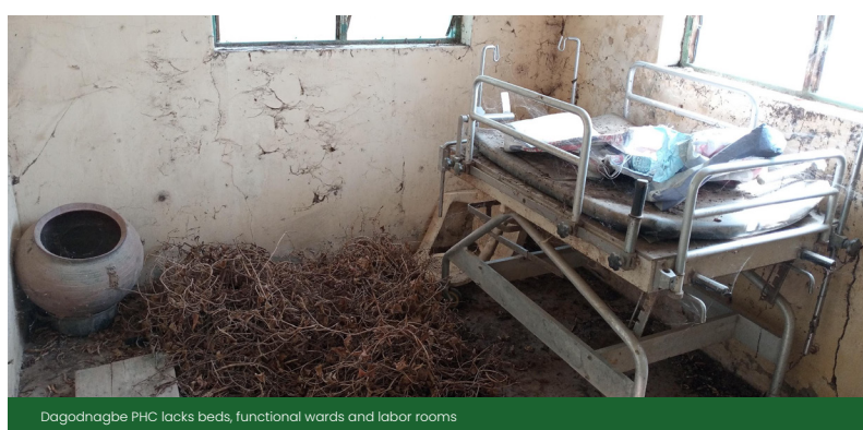
Dagodnagbe PHC lacks beds, functional wards and labor rooms
