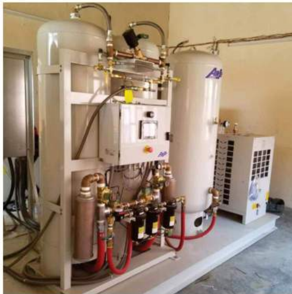
The new medical gas plant
