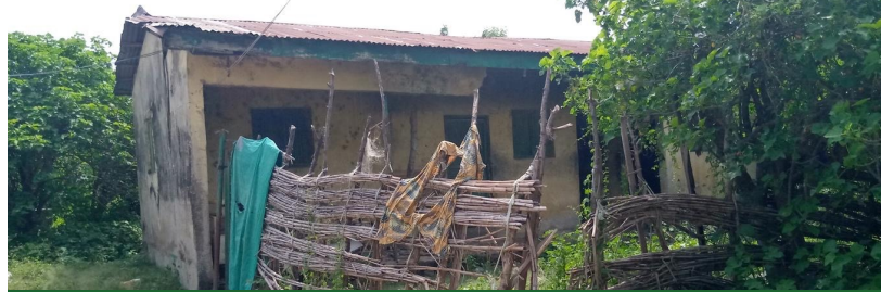
Gwarjiko PHC has a staff quarter, which is rare in PHCs in Nigeria. However, the quarters need repair themselves
