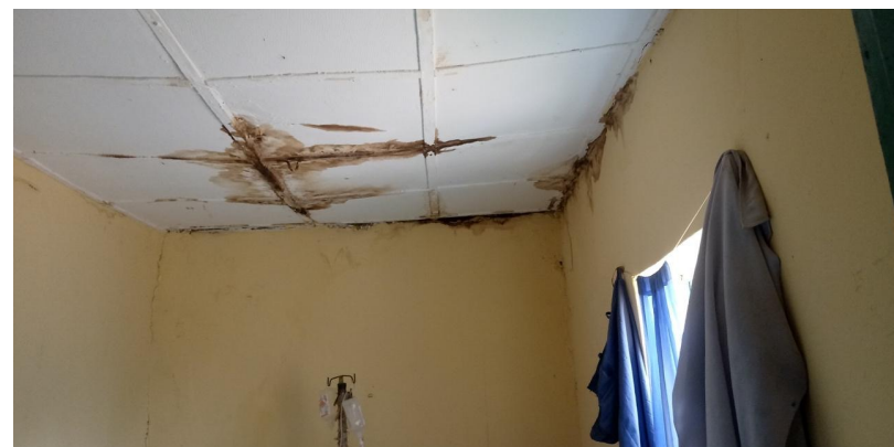
Among many other challenges, Gwarjiko PHC suffers from broken ceiling
