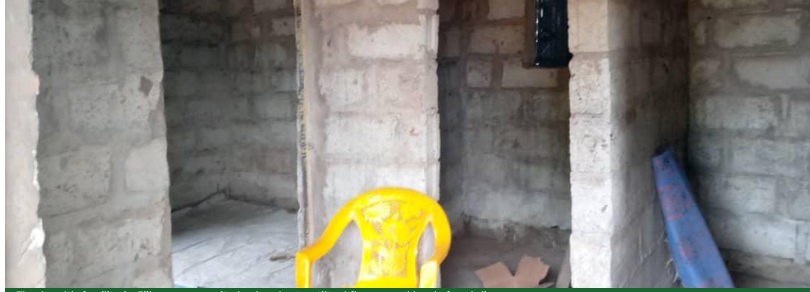
The health facility in Ejiko community lacks plaster, tilted floors and beds for delivery
