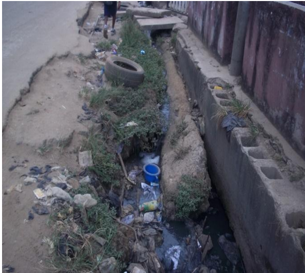
Figure 4: Showing a poorly maintained drain
