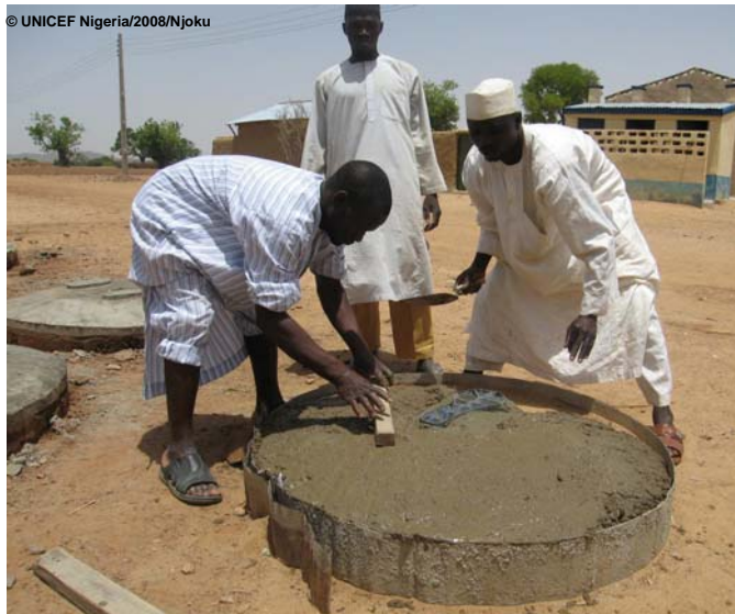
Local artisans constructing sanitation platforms for VIP latrines in Kadadaba village, Maru Local Government Area of Zamfara. These artisans receive training as part of the support from the Federal Government and UNICEF's WASH programme
