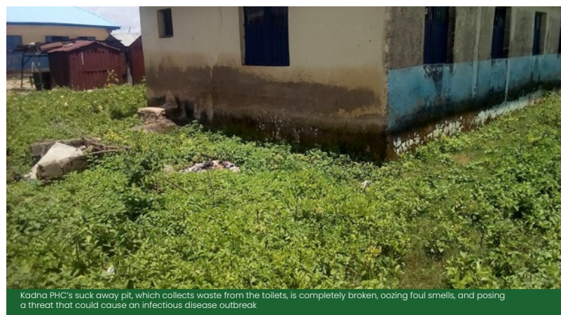
Kadna PHC does not have a proper waste disposal site, and waste are disposed off in the facility premises
