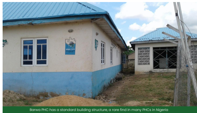
Barwa PHC has a standard building structure, a rare find in many PHCs in Nigeria
